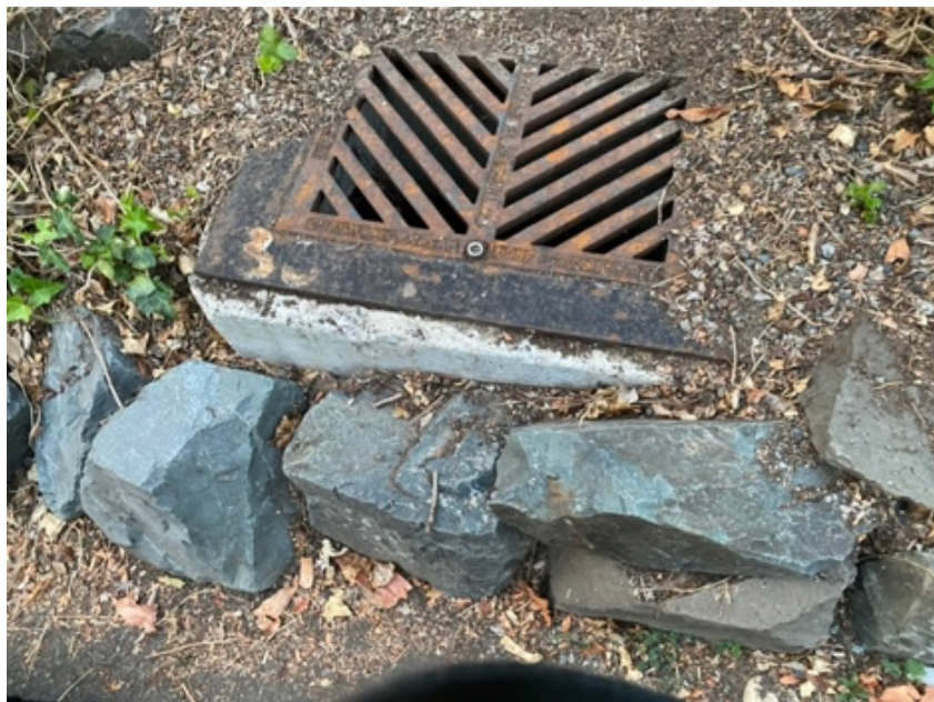
Photo of elevated catch basin on Maker Street (same culvert referred to per Photo 3 in Storm Drainage Report).
