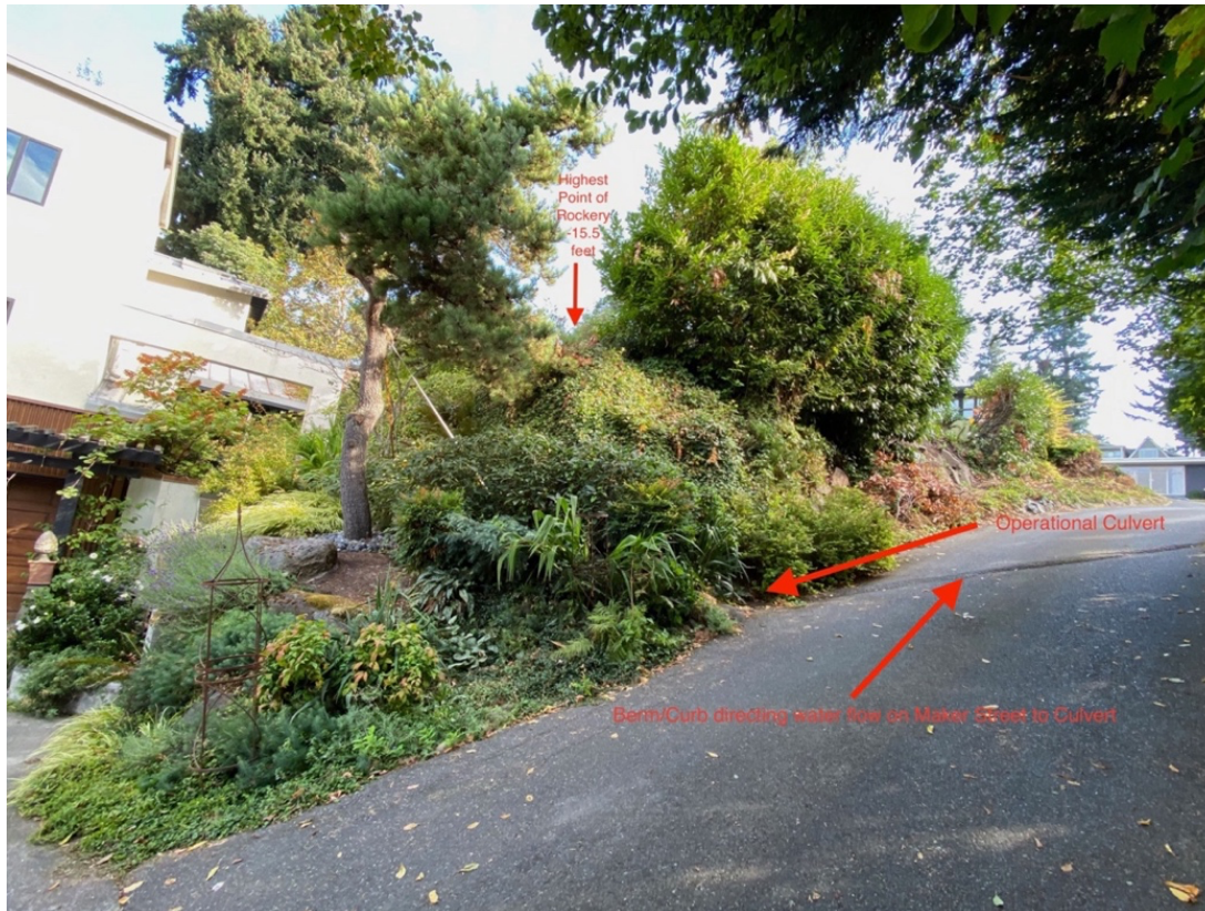
Photo of Maker Street: Looking up from house on 7030 Maker Street to adjacent uphill property, 6950 SE Maker Street. Arrows point to operational culvert and berm/curb that directs Maker Street runoff to culvert.
